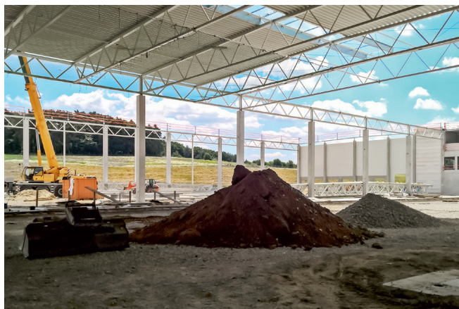
Sites close to our customers: The construction of the new Holledau corrugated cardboard plant in Bavaria.
